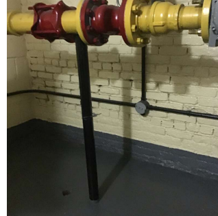
Gas Meter Room
